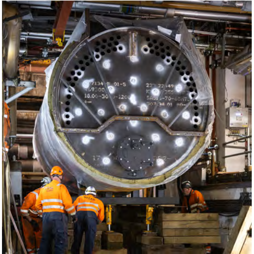
Right: Installation of the new boilers as part of the removal of central steam generation on the South Kensington Campus.
