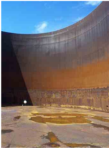
Figure 2.2: Photograph of a large oil tank that is assembled by many large slightly curved plates.
